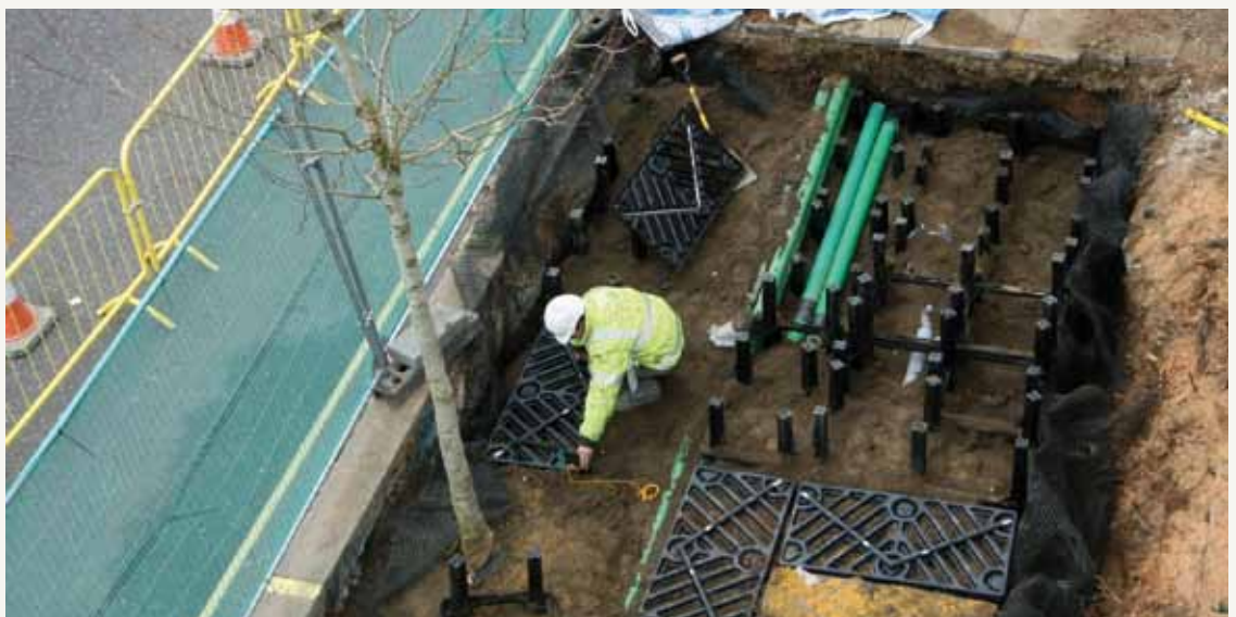
Installation of the 'Silva Cell' modular cell system ensuring news street trees planted in front of the new RAF Bomber Command Memorial in London will grow big. © Jeremy Barrell
