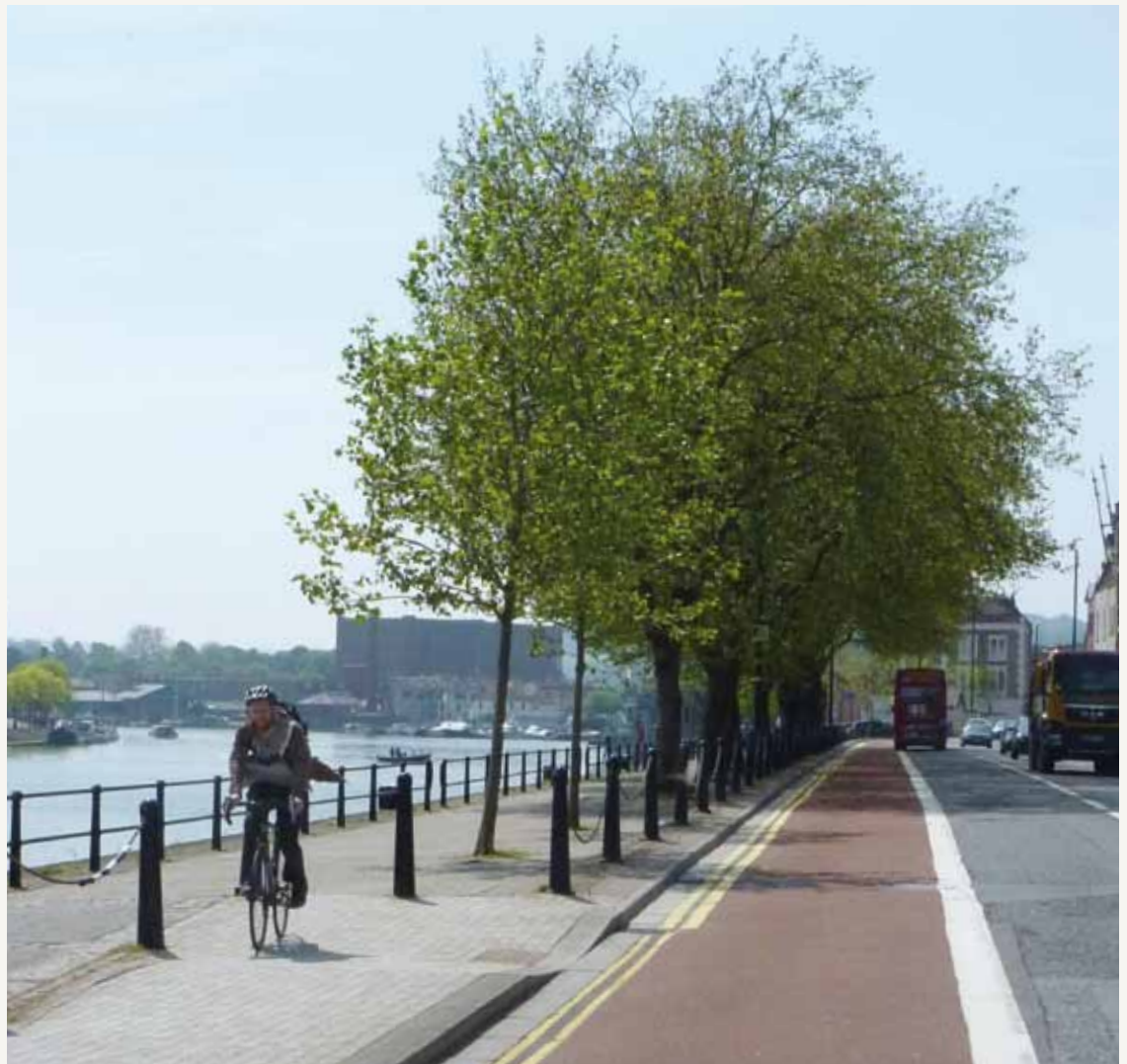
Replacement trees next to where an underground stormwater storage tank was installed by Wessex Water. © TreeBristol
