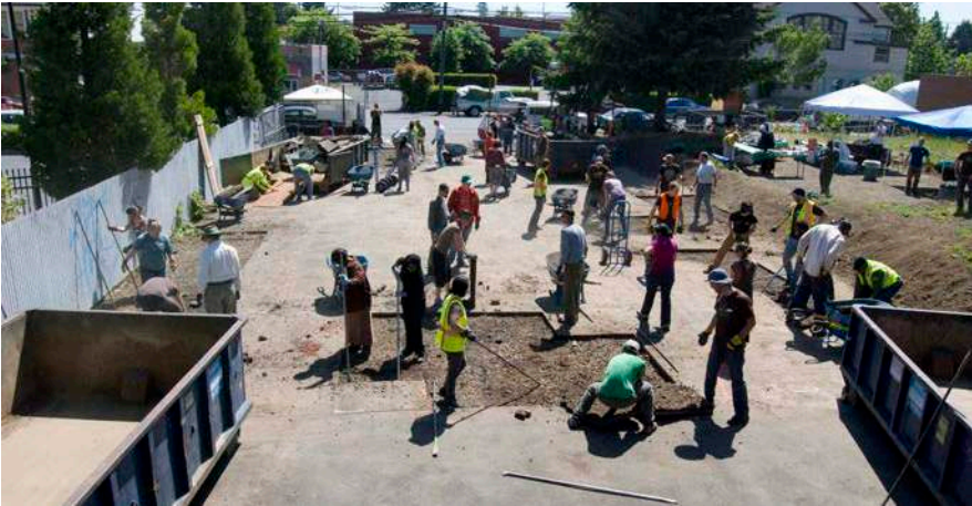
In Portland, US, nonprofit organisation Depave promotes the removal of unnecessary concrete pavement.
